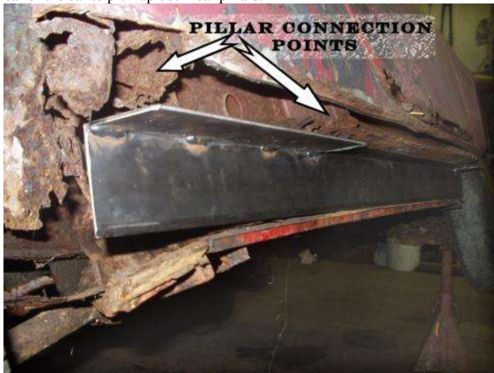
Landing spots for the non-existent rear pillars
